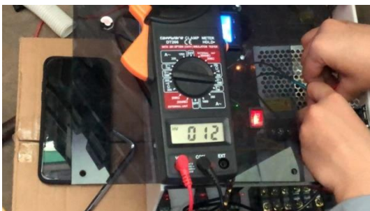
Gambar 8. Pengukuran Power Supply
